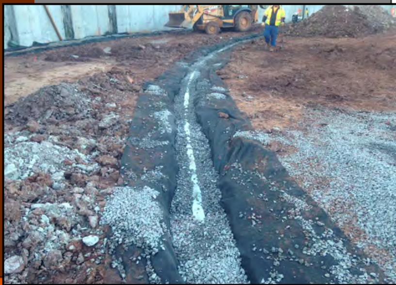
PICTURED LEFT: UNDERGROUND DRAINAGE SYSTEM
