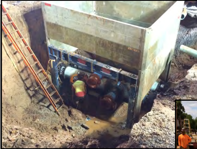
Pictured Left: New pipe and valves to new chilled water lines running east
