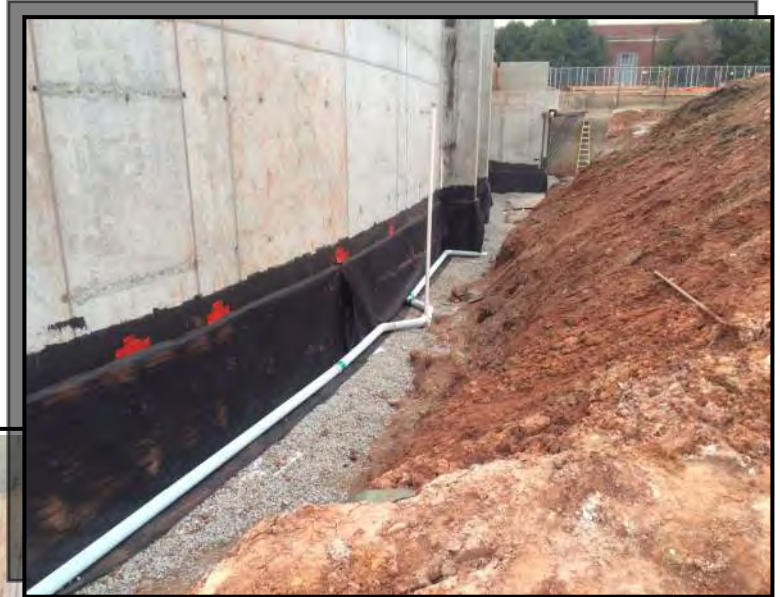
PICTURED LEFT & BELOW: UNDERGROUND DRAINAGE SYSTEM ON EXTERIOR OF BUILDING IS INSTALLED
