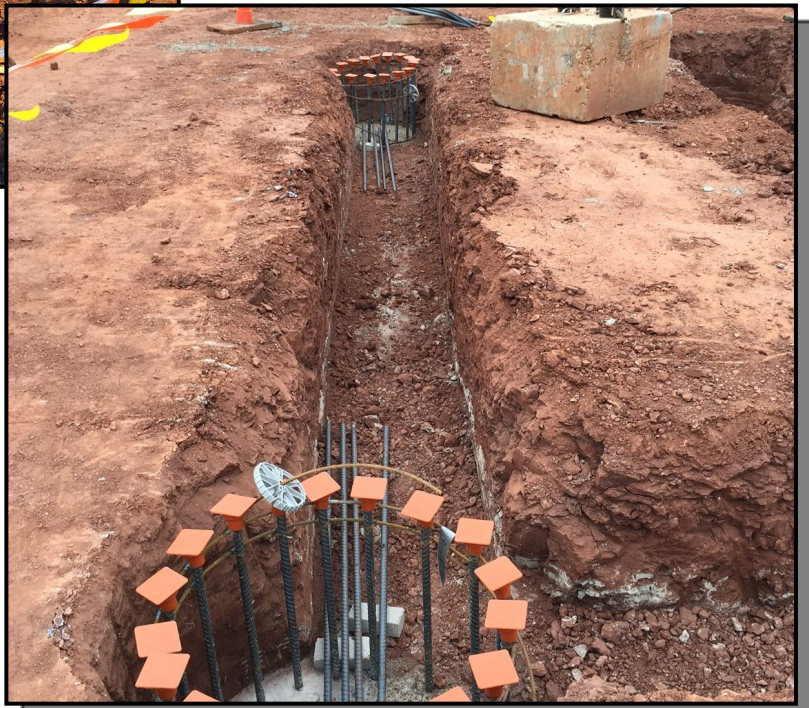
PICTURED ABOVE AND RIGHT: EXCAVATED GRADE BEAMS AROUND STAIRS AT NORTH HALF OF BUILDING
